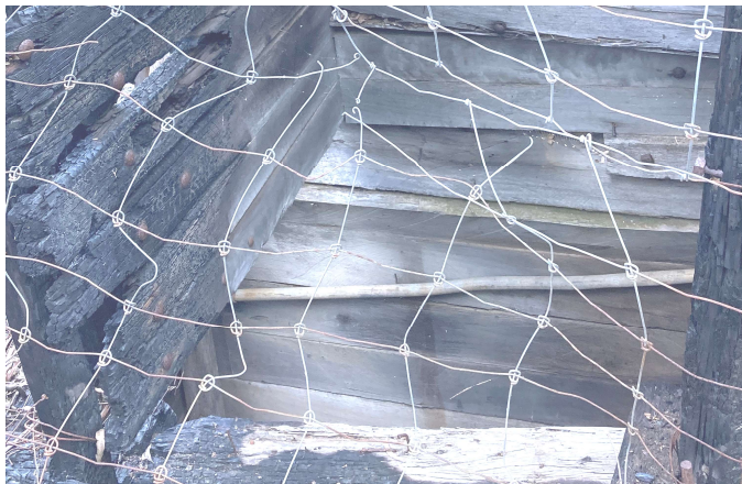
Plate 2: Main shaft (2m by 1.2m) at surface with sound timbers below ground level
